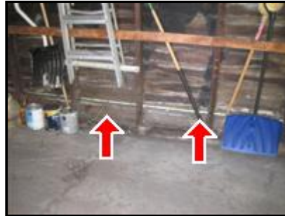
B. Picture 1 Gaps in siding
